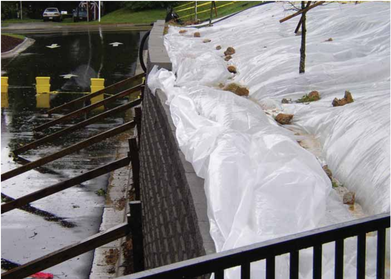
Photo 10 | Poor surface drainage infiltrates reinforced soil.
