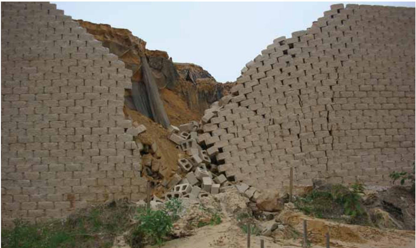
Photo 3 | Inadequate surface-water control during work.
