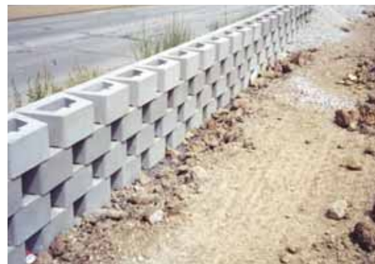
Photo 8 | Loose soil left near drainage aggregate.
