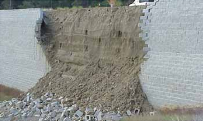
Photo 6 | No compaction within 3-5 feet of wall face.
