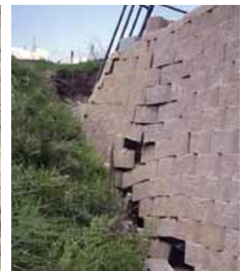
Photo 9 | Surface water erosion of completed structure.
