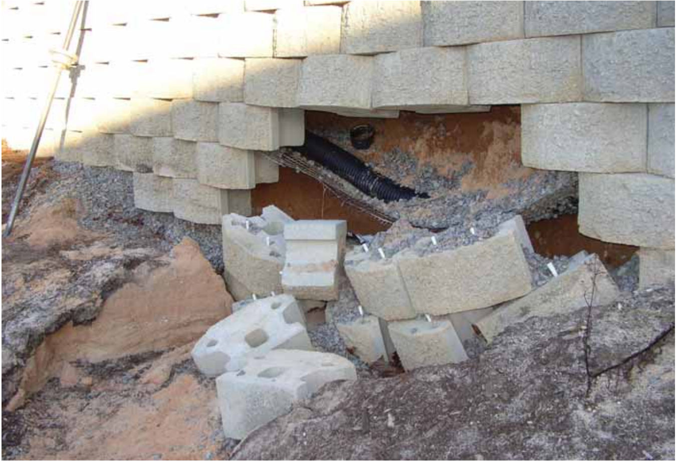
Photo 4 | No outlet provided; collection pipe above flow line.
